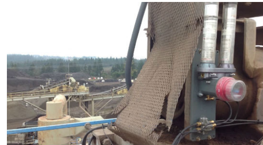
Titan II conveyor lubrication
